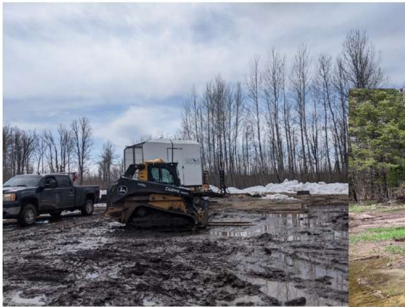
Rutting and damage (DNR April 2023)
