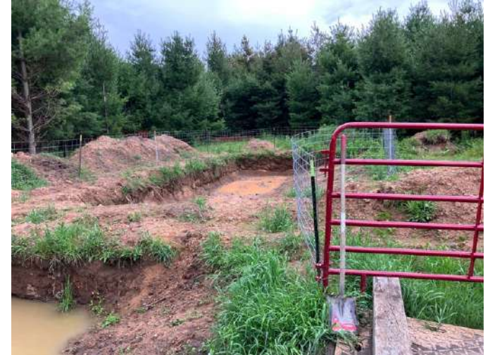
Unlined sump in wetlands, mat corner (DNR 2024)
